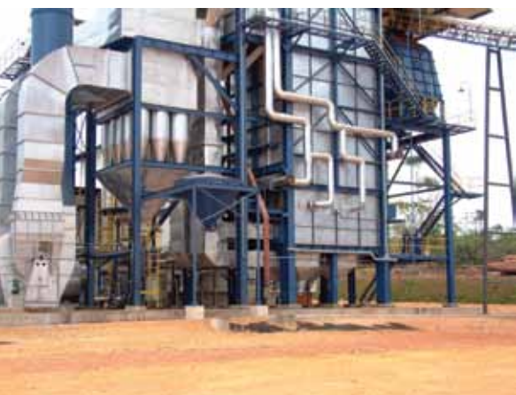
Photo 10.1. A wood-fuelled power station was built at the sawmill site in Itacoatiara. (Photo N.R. De Graaf)
